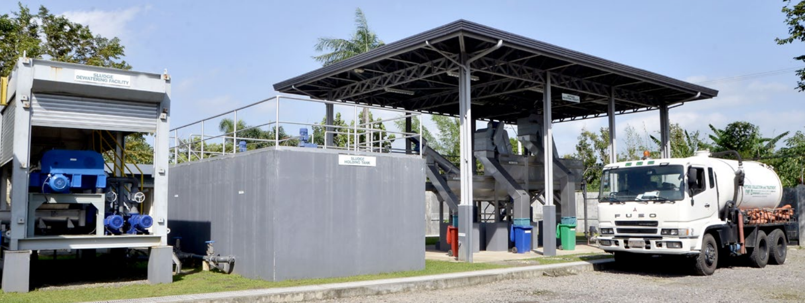
Photo shows Environkonsult's sludge dewatering facility, sludge holding tank, septage receiving facility, and desludging truck.
