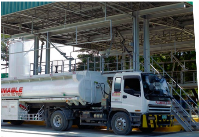
Tank truck loading facility
